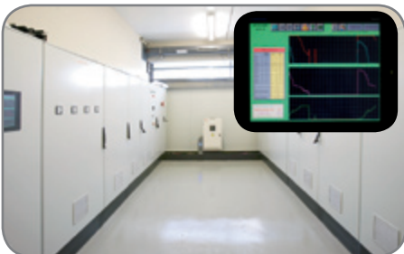
Electrical control cabinets
